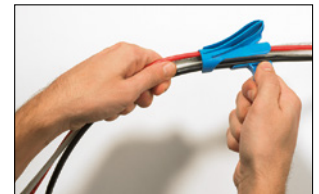
Insert one or more cables into the insertion slot of the applicator tool.
