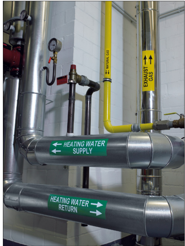
Large and highly visible pipe marking.
