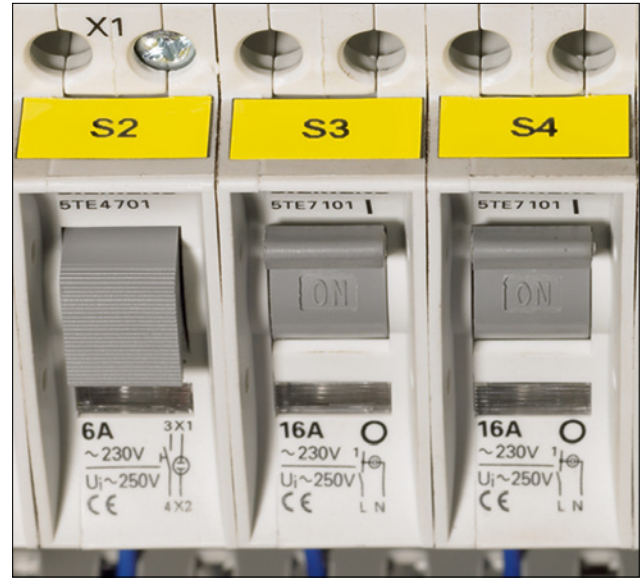
Clearly identified labels ensure easy network wire and cable management.
